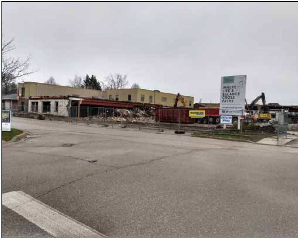
The former Magnesun Furniture, a longstanding New Hamburg business, was demolished recently to make way for Cassel Crossing, a 62-unit townhouse development. Photo by Sharon Leis
