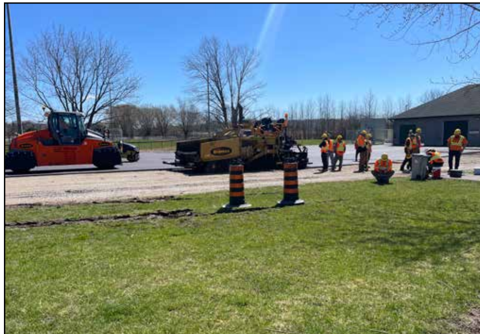
Paving crews with Brantco are seen finishing paving the parking lot on Monday at the Shakespeare Optimist Hall. Photo by Gary West
