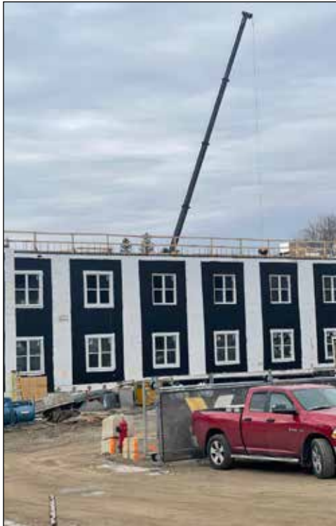
A large crane is seen recently, placing pre-fab roof slabs, built by Oxford County's Stubbe's Pre-Cast of Norwich, into the new People Care long term care home in Tavistock. Photo by Gary West
