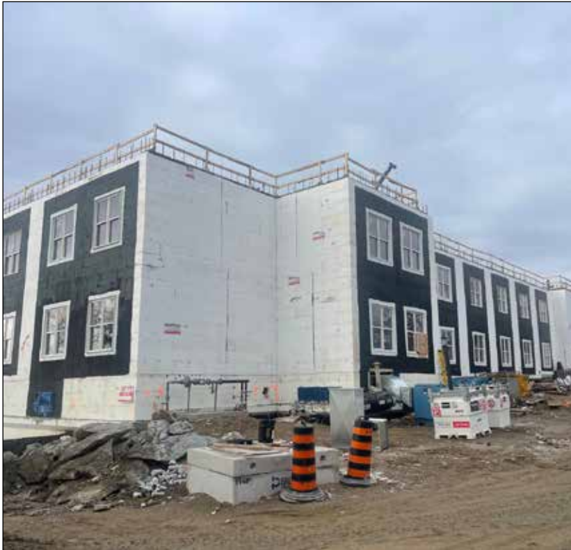
A view from the south of the construction site at the new home of People Care long term care in Tavistock being built by Van Del Construction, which is celebrating its 50th year in business this year. Photo by Gary West
