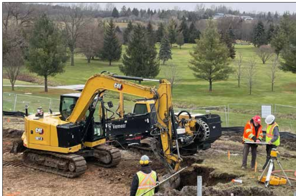
Paul Bender of MTH Contracting (in orange jacket) is pictured above discussing the site plan for the Penrose Suite development at St. Marys Golf & Country Club on Tuesday, December 5. (Stewart Grant photo)
