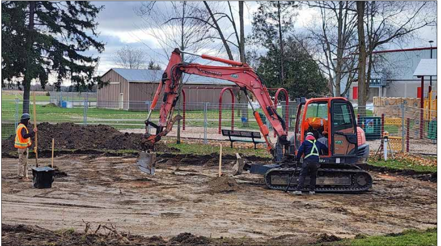
Construction on Tavistock's Spray Pad started this week. Excavating is the first step before plumbing can be roughed in to ready for a concrete pour. It is expected to be operational in the summer of 2024.
