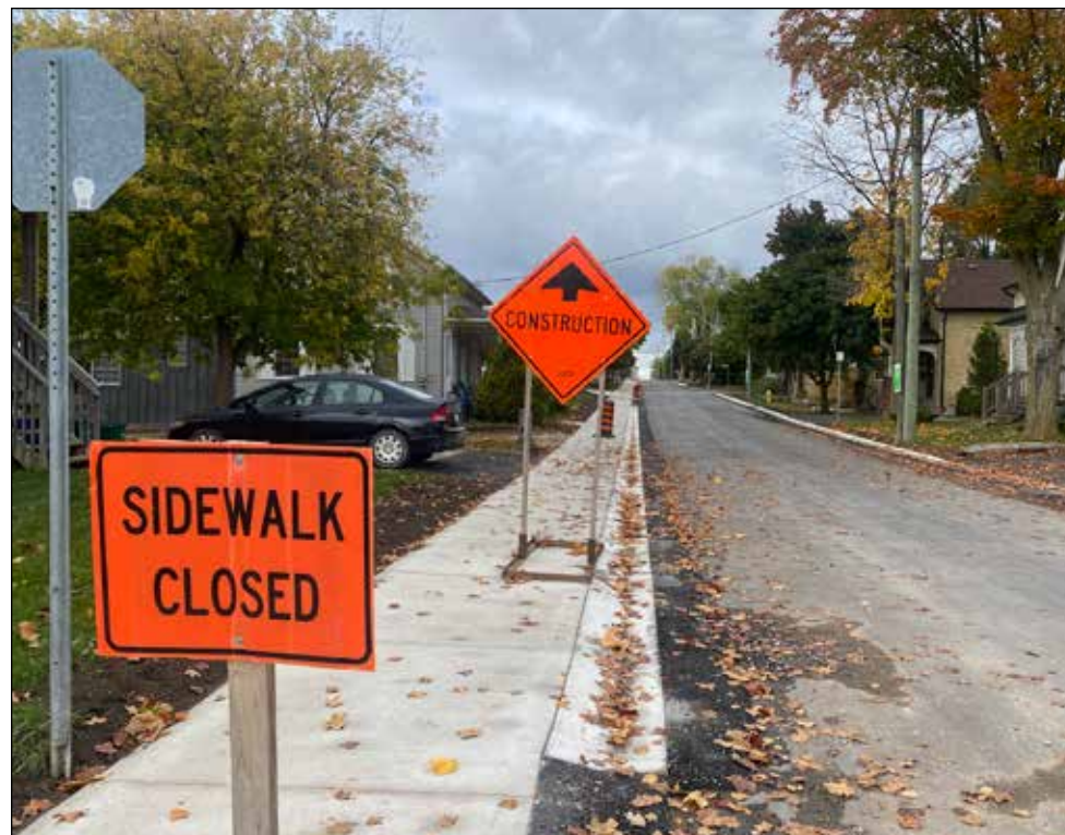
Queen's Bush Road and Molesworth Street in Wellesley village have reopened to traffic in both directions after the first phase of the Queen's Bush Road reconstruction project is complete. New asphalt has been installed on both streets, along with concrete curbs. Sidewalks appear to be completed, with a "Sidewalk Closed" sign still up on Molesworth as of Saturday, October 14. There will be two more phases of the Queen's Bush Road reconstruction project, taking place in 2024 and 2025. (Photo credit: Veronica Reiner)
