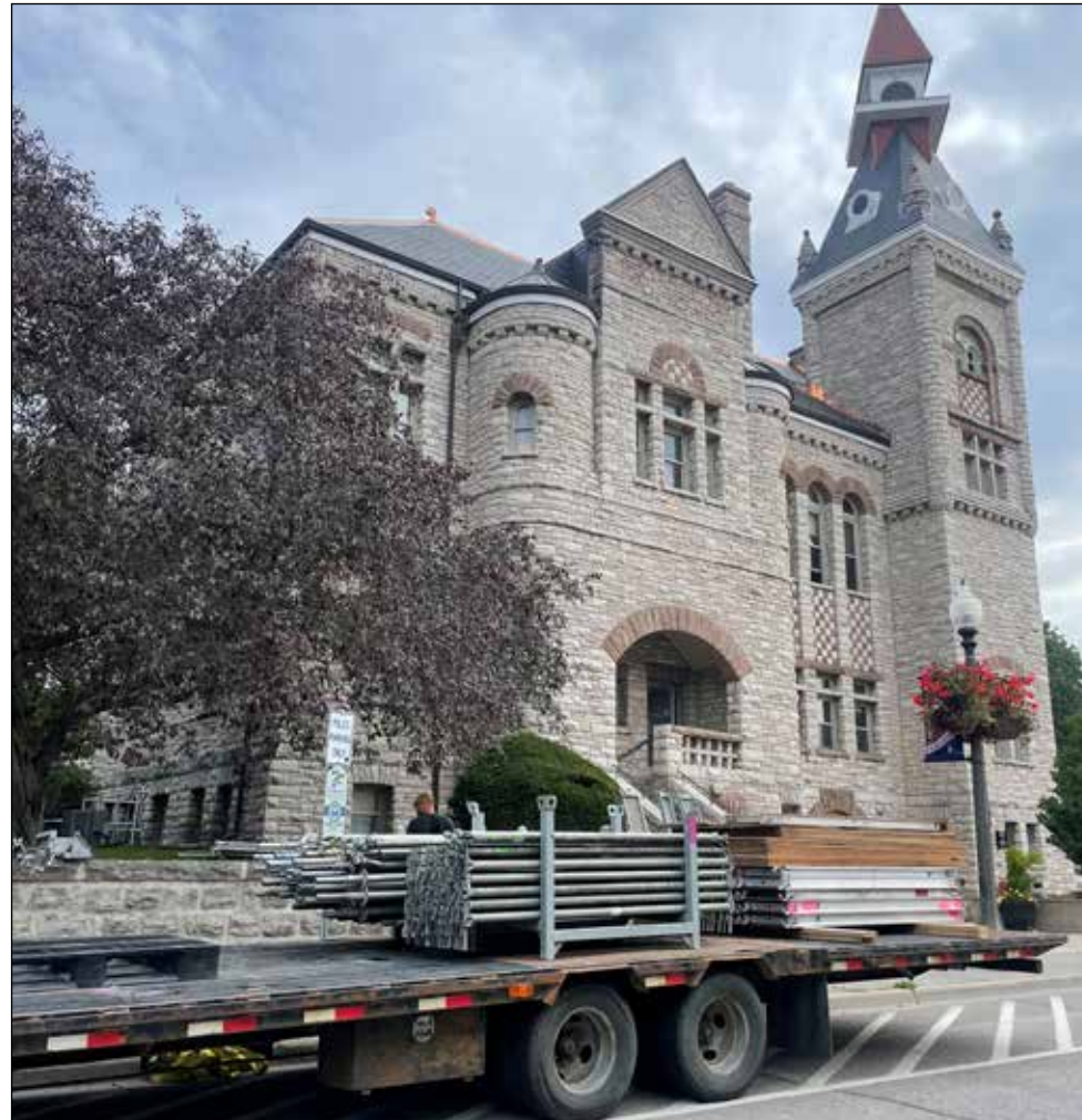
The final pieces of scaffolding were loaded up and taken away on September 25th following Robertson Restorations' completion of the Town Hall slate roof replacement project. (Stewart Grant photo)
