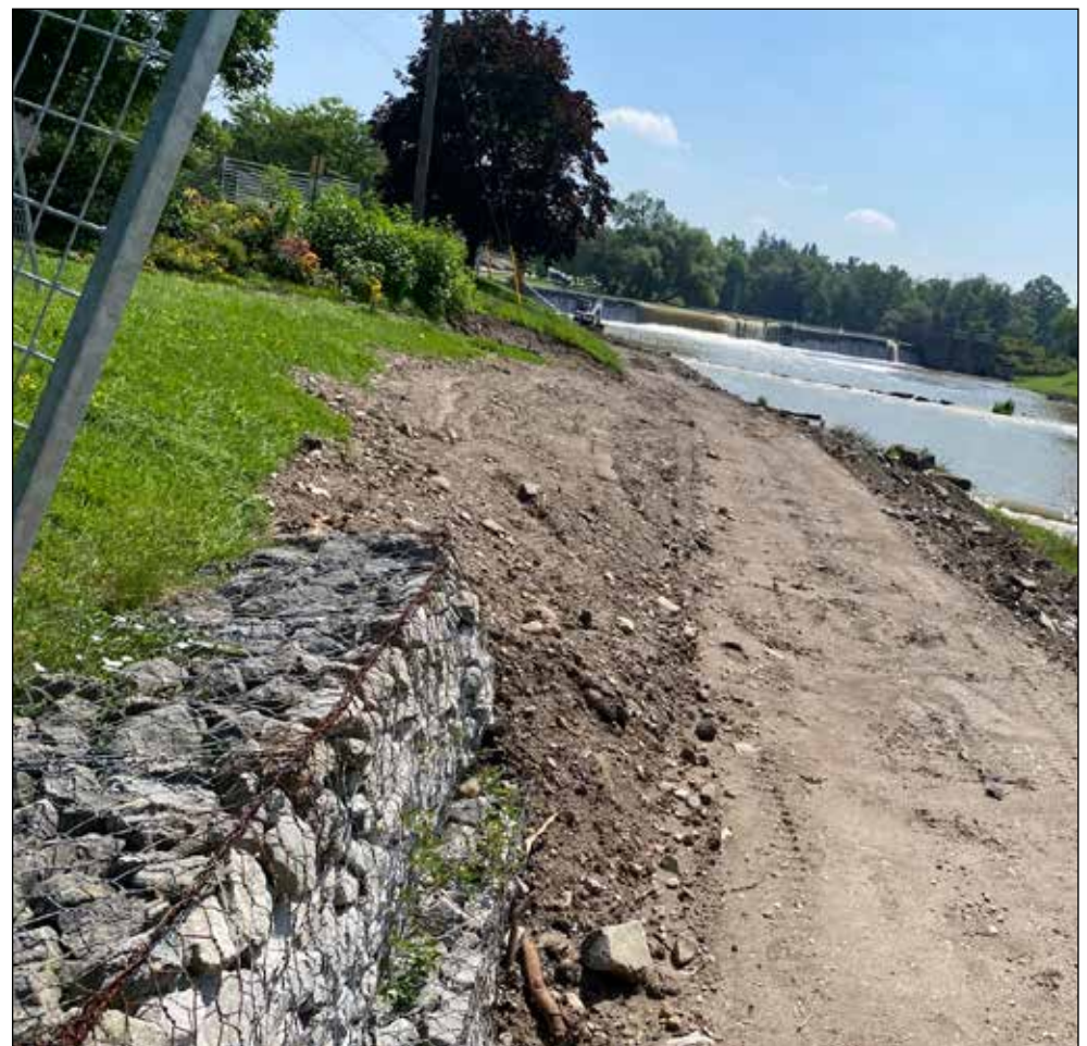
Construction is currently underway for the Nith River Promenade. The contract, which was awarded to Lyncon Construction Inc. in May, includes trail and lighting enhancements. There is no public access during the construction period, and the project is expected to be completed by October 30. (Photo credit: Veronica Reiner)
