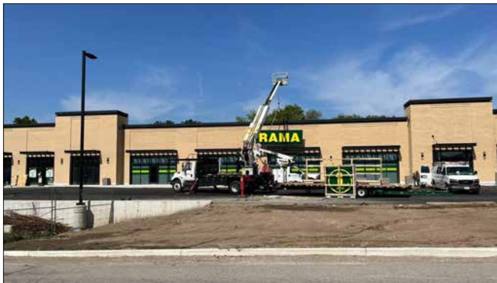
The Union Street plaza construction is coming along, with the Dollarama sign being constructed. The Dollarama will be the largest sized business in the plaza, which will also include a City Pizza, BarBurrito and Tumeric. (Photo credit: Susan Hammer)
