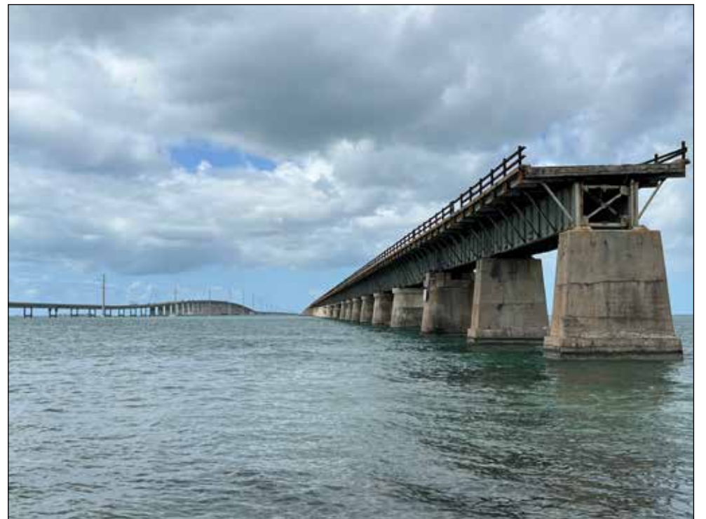
A section of the railroad that remains – with Highway 1, which sometimes used the railway bridges, shown to the left.
