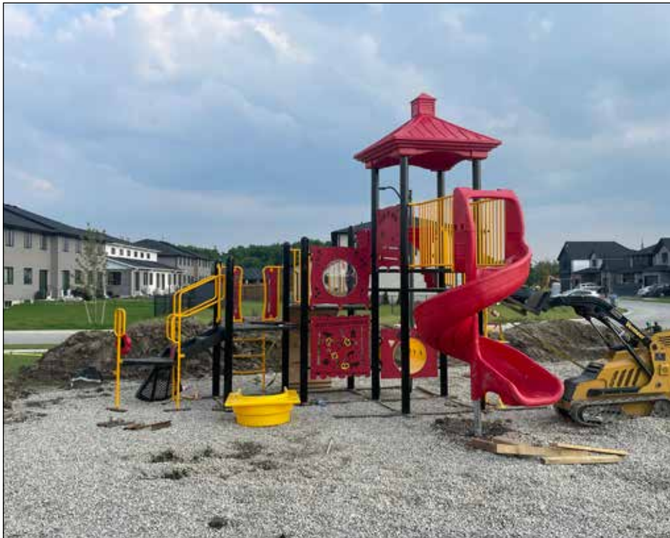
On Monday, July 17, the brand-new playground set within the Trailside/Hooper development was largely put together. Some additional installation remains, but it won't be long before neighbourhood children are able to enjoy this new structure. (Stewart Grant photo)
