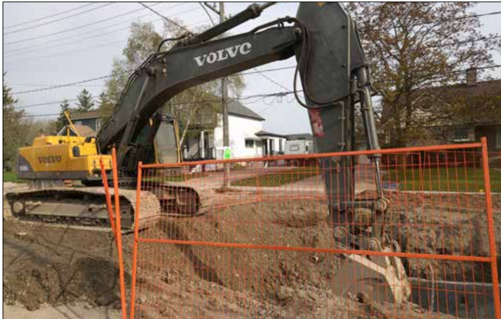
The reconstruction of Snyder's Road East in Baden as of Friday, May 12. (Photo credit: Veronica Reiner)
