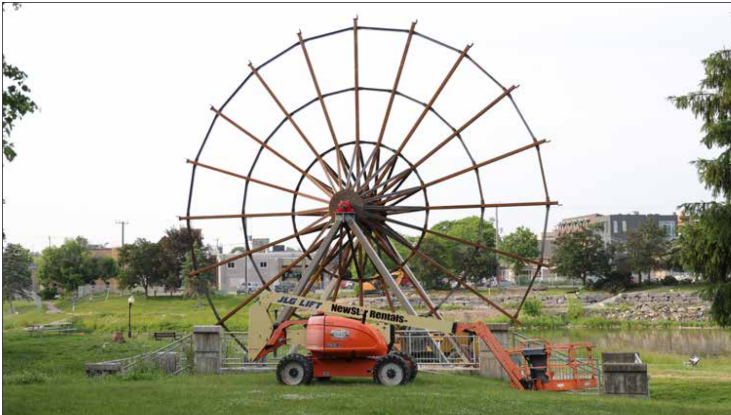
The New Hamburg steel waterwheel up as of Monday, June 19. Buckets have since been installed on the structure, with work being done by Iron Bridge Fabrication.
