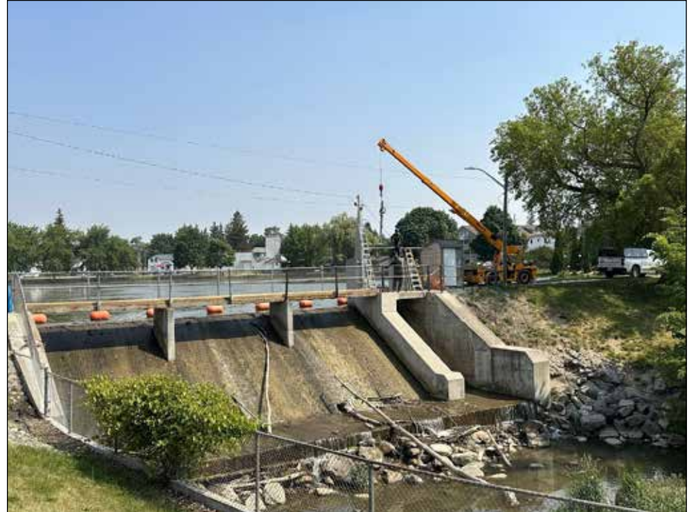
The Grand River Conservation Authority began making improvements to the gate on the dam at the Wellesley pond the week of June 8. They will be working there until around July 8. (Photo credit: Township of Wellesley)
