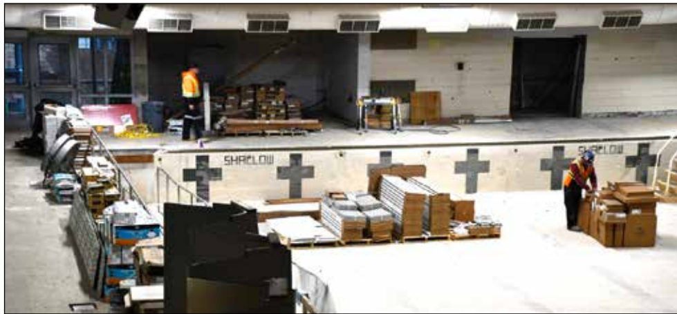
Workers have been busy working to complete the tiling on the pool deck. Once the pool is open, programs will resume. Along with the pool, there is a new second floor meeting room, a barrier-free pool viewing area, a health club addition and a new customer service base.
