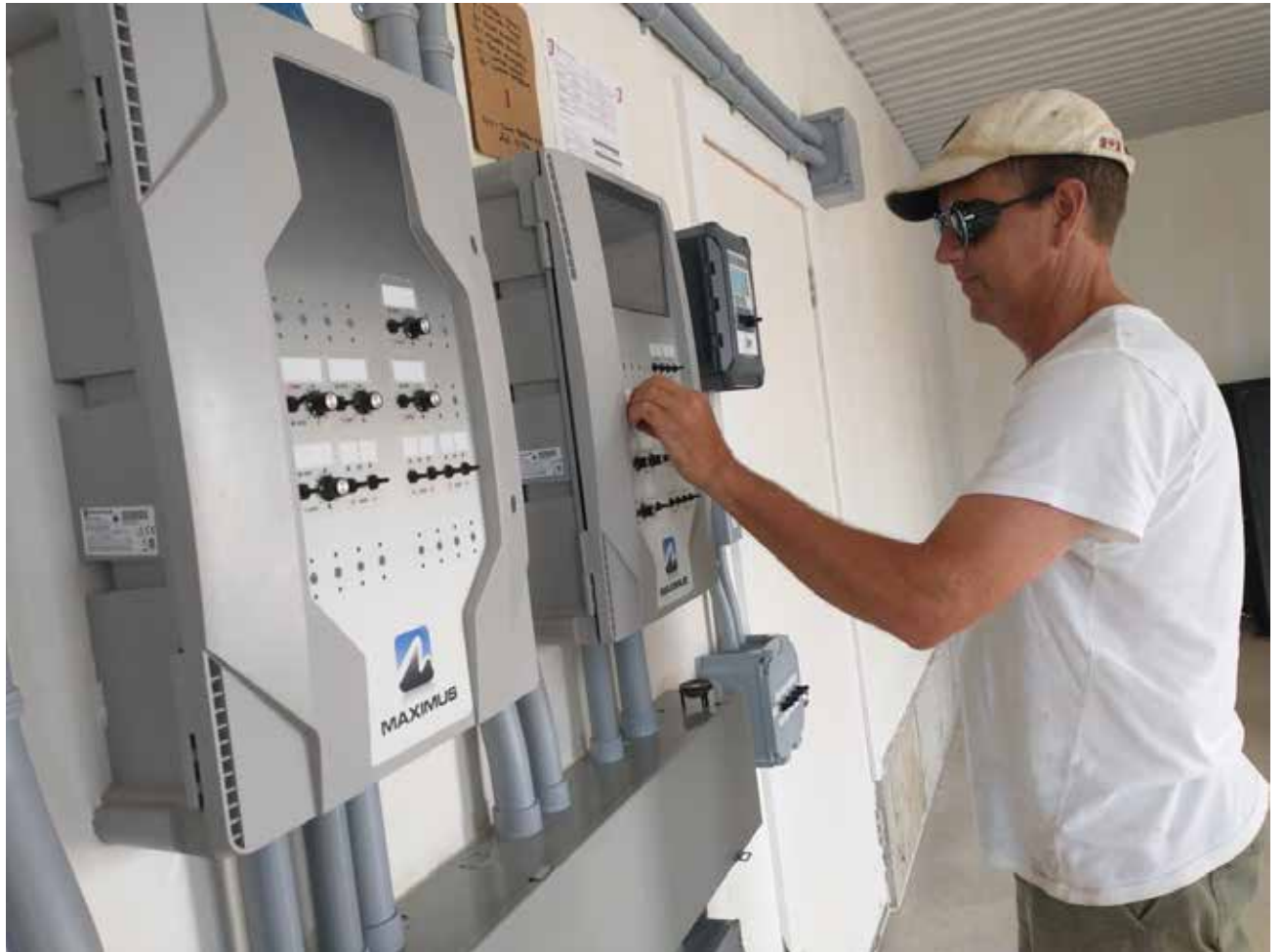
Bruce Van Der Molen uses a single control system to maintain the building’s mechanical systems.
