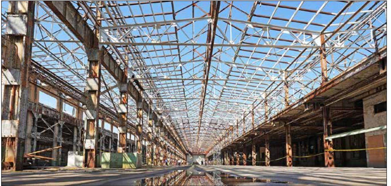
The interior of the Grand Trunk building, part of an 18-acre rejuvenation project the City of Stratford has undertaken. As seen in the photo, the lack of a roof may prove to be a significant barrier, according to consultant Joe Svec. (CONTRIBUTED PHOTO)
