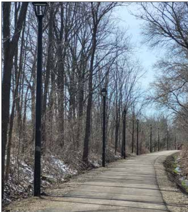
A total of 23 light standards are currently being installed along a recently improved section of the Grand Trunk Trail in St. Marys. Photo by Wendy Lamond
