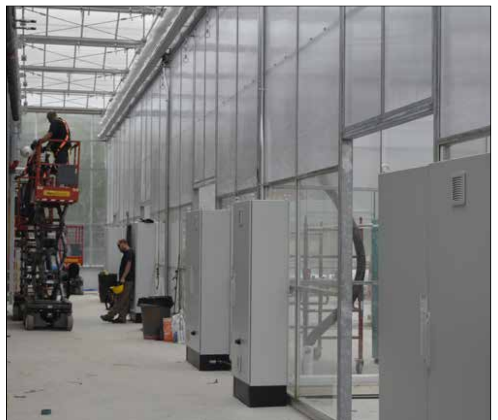
Five bays in the greenhouse will allow staff to control conditions such as temperature and humidity to get the best research data possible.
