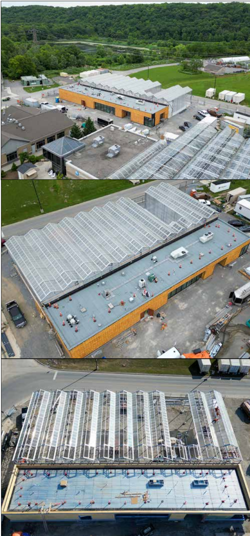
Drone shots of construction at the new research greenhouse on Niagara College's Daniel J. Patterson campus in Niagara-on-the-Lake. ~ Niagara College photos
