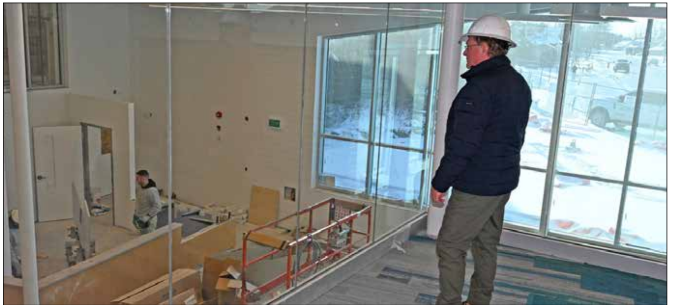
COMMUNITY CENTRE CONSTRUCTION CONTINUES (JEFF HELSDON PHOTO) Chris Baird, project manager for the Tillsonburg Community Centre and pool renovations, overlooks the new customer service area from a newly-created glassed-in meeting room. The construction company will turn the facility back over to the town on Jan. 31. After cleaning, filling the pool and many other tasks, the goal is to have people in the water by the third week in February. Story below.
