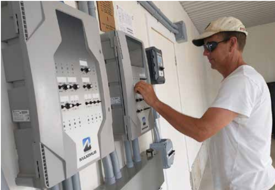
Bruce Van Der Molen uses a single control system to maintain the building’s mechanical systems.
