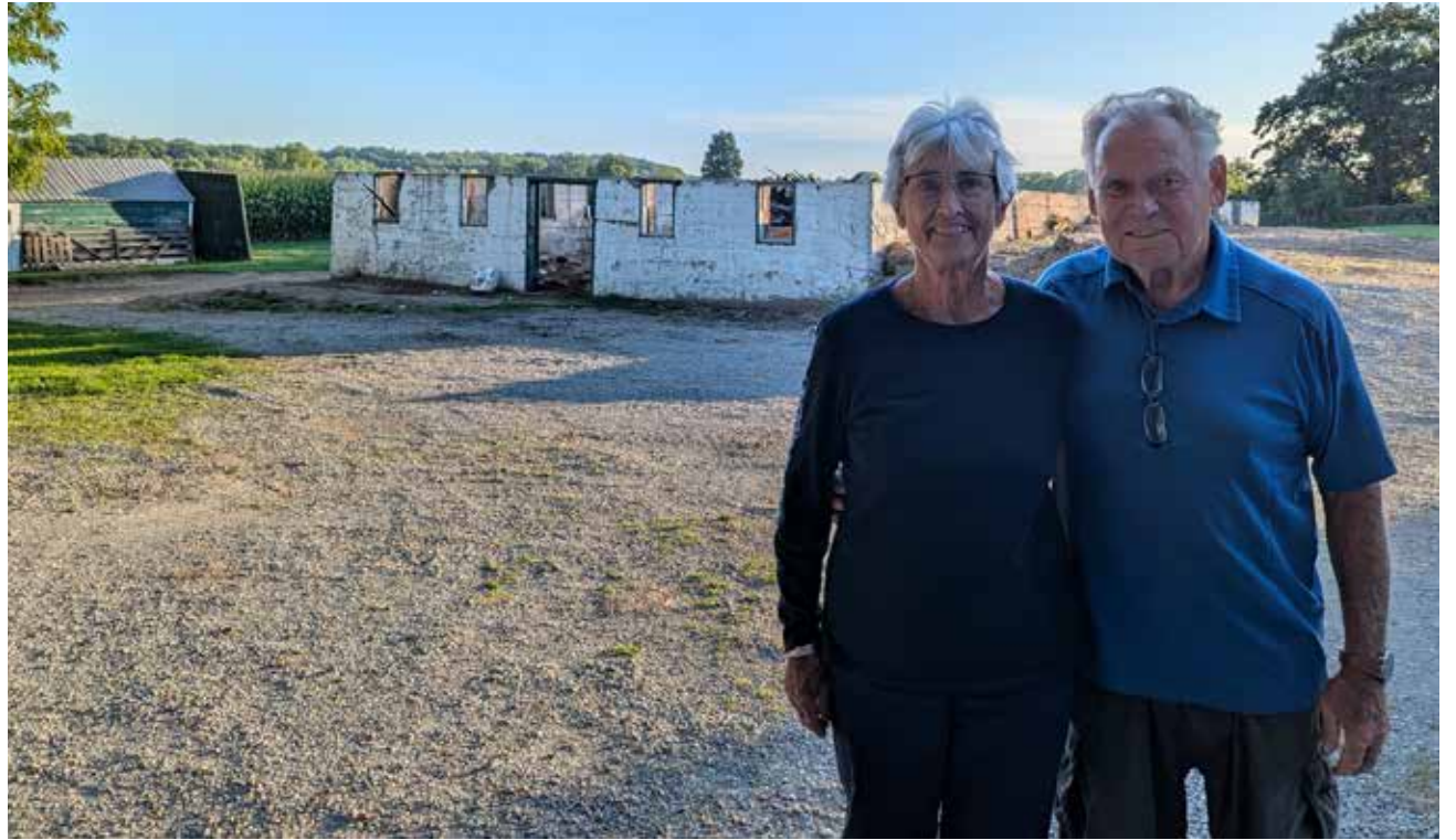
It took less than a week for the crew to remove the historic barn from Lois B. and Don Douglas' farm on Highway 54 near Brant County 22. Now the old structure is gone, a second living space – a 'barndominium' – will be build there instead so one of their daughters and her husband can live on the farm as well.
