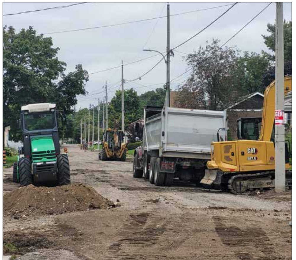
This year's reconstruction of Wellington Street South from Park Street to St. Maria Street and the reconstruction of Victoria Street from Church Street South to Water Street South officially got underway on Aug. 12. Photo by Wendy Lamond
