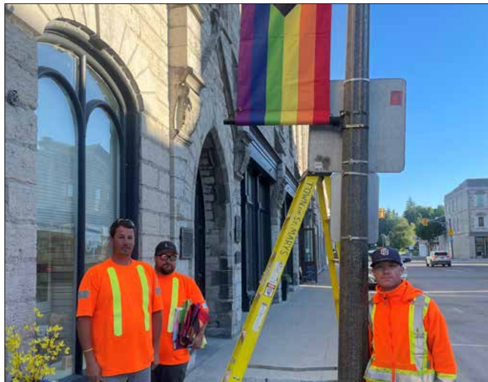
Town of St. Marys employees Kenny Hutton, Alex Taylor, and John Hahn were at work early in the morning on Friday, May 31 installing colourful Pride banners on light stands throughout the downtown. Approximately 30 banners have been installed again this year in recognition of Pride Month. Photo by Stewart Grant
