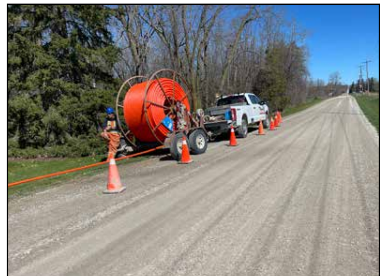
Steve Pilon from Wingham rolls out the orange plastic tubing in which the fibre-optic wire will be placed by another machine. Photo by Gary West
