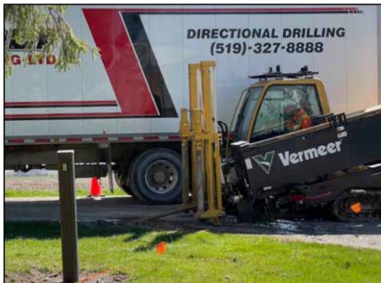
Ben Rheubottom from Walkerton operates the Vermeer bidirectional drilling machine April 22 for Weber Contracting Ltd. On Perth Road 106 in South Easthope Township. Photo by Gary West
