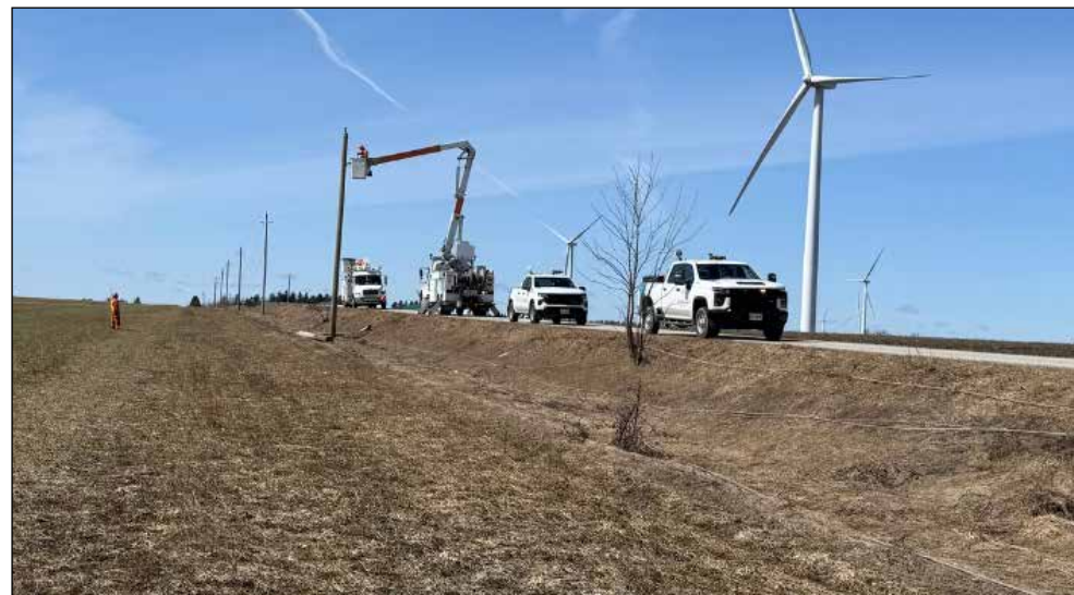
Crews working on downed power lines in the Highway 124 area, north of Shelbourne.
