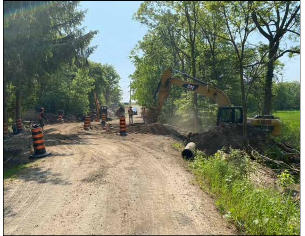
The contractor operating without proper erosion and sediment controls. (All photos by Courtney Huber)
