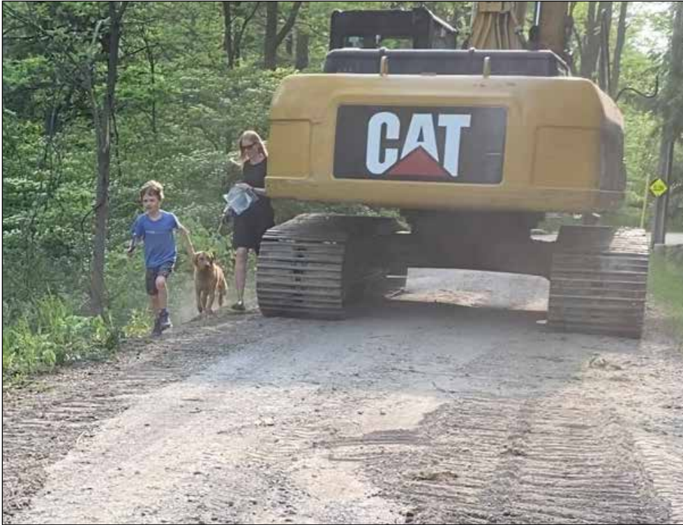
A New Dundee resident walking her son to the end of Cottage Lane to get on the bus. The contractor was operating on the road, with the excavator blocking the one way lane. There was no flagger to direct the family across from the construction site safely.
