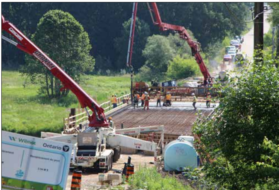
Workers began to pour bridge deck for the Bridge Street bridge replacement project on Wednesday, June 21. The project was awarded to Sierra Bridge Inc. of Woodstock for $4,782,267.90 during a council meeting in June 2022. (Photo credit: Anne Loeffler)
